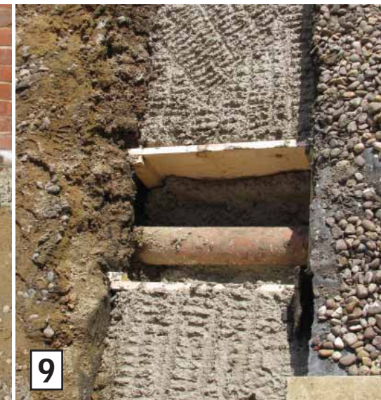
Any drainage pipes will be identified, protected and 'bridged' by concrete lintels.
