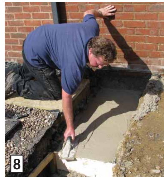
The concrete is floated to form a level surface area to build upon.
